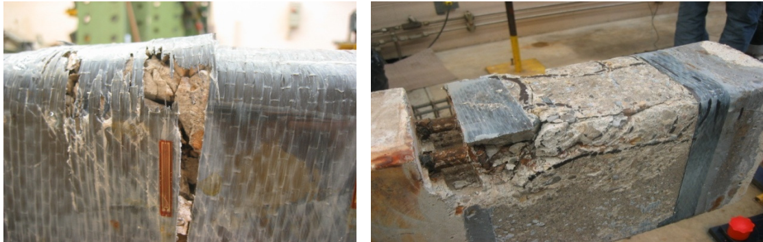
a) CFRP failure b) Splitting concrete cracks Figure 3. Bond failure of the wrapped corroded beams (Groups W5 and W9).
